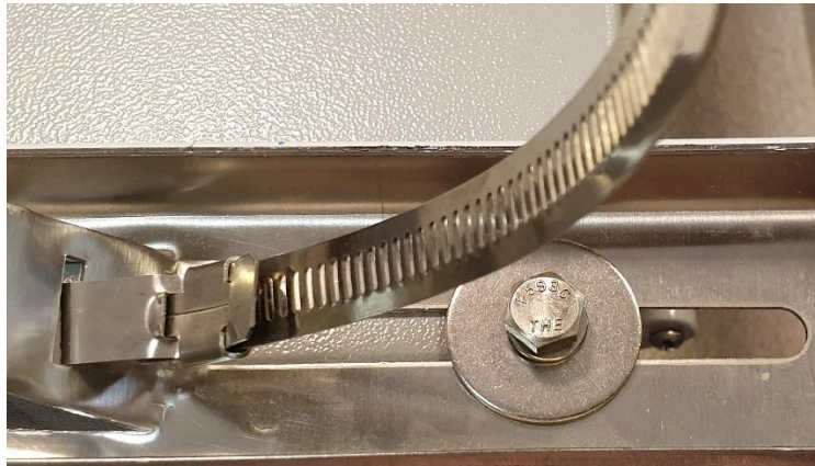
Figure 13: Close-up of washer on pole mount
